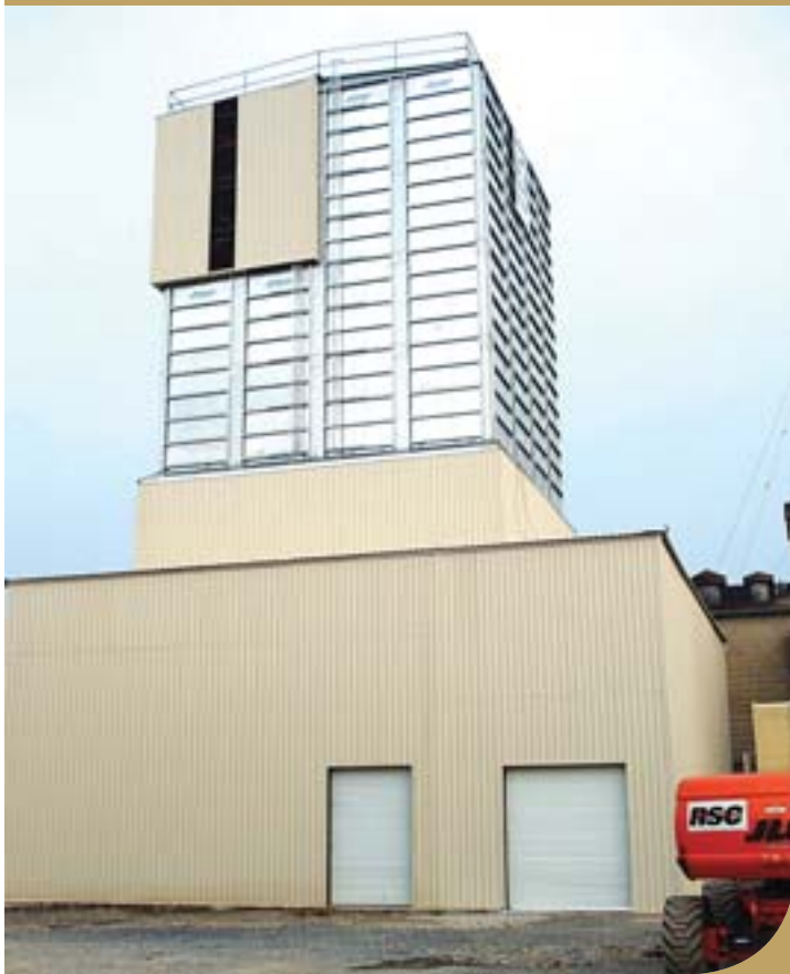
Photo: Ridley's Equine Business Unit is building an all-equine feed facility in Chambersburg, Pennsylvania to serve the growing equine market in the Mid-Atlantic region.
